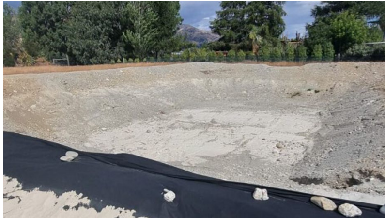
A sediment basin may be proposed as an alternative to an SRP for gravelly ground with high infiltration rates. Provide evidence of high infiltration rates and continue to monitor this — as infiltration can decrease over time as silty fines accumulate in between pores.
