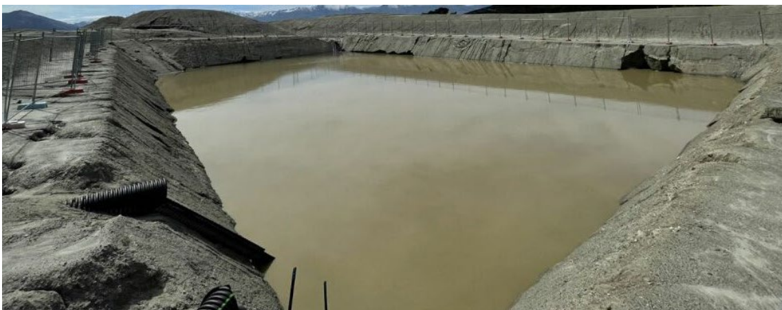
Large offline storage pond constructed to manage extreme rain events, in addition to multiple SRPs across this large earthwork site, providing resilience during calamity situations.
