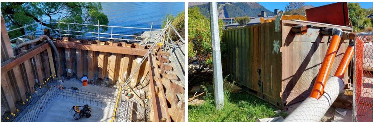
Cofferd dam in place to allow construction of a stormwater outlet (left), with dewatered water treated in a settlement tank before being discharged back to the lake (right)
