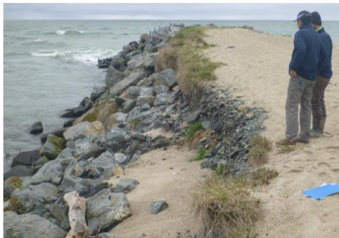
Figure 2.8: Koau River Mouth training wall (north) following a storm when it was badly damaged by the removal of rip rap by high sea levels and large waves, exposing the training line to further damage (Bloor, 2017).
