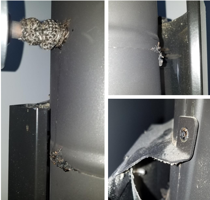
Figure 21 Household 1 Flue Showing Build-up of Creosote
