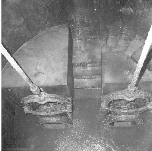
Photo Four: View of Sluice Valves inside the Intake Tower
