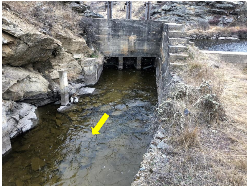
Photo Six: View of Outlet Gates at Upper Bonanza Weir and the start of the Upper Bonanza Open Channel Race
