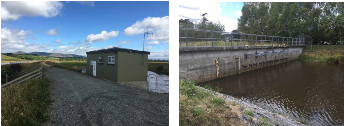
Figure 2: Paretai pump station and floodbank (left) and Kaitangata locks (right) on 23 January 2017. The station, locks and floodbank are part of the Lower Clutha Flood Protection and Drainage Scheme
