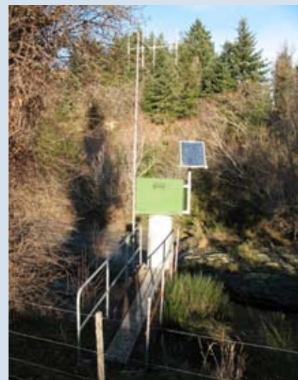
Hydrological monitoring station on the Shag River at the Grange
