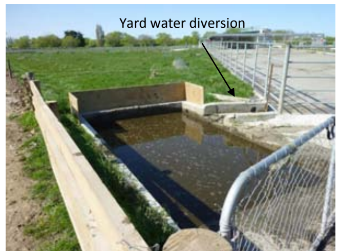
After: Extra height on stone trap so doesn't overflow when cleaning with a digger, drain removed so no overflow can enter a waterway. Yard diversion installed.
