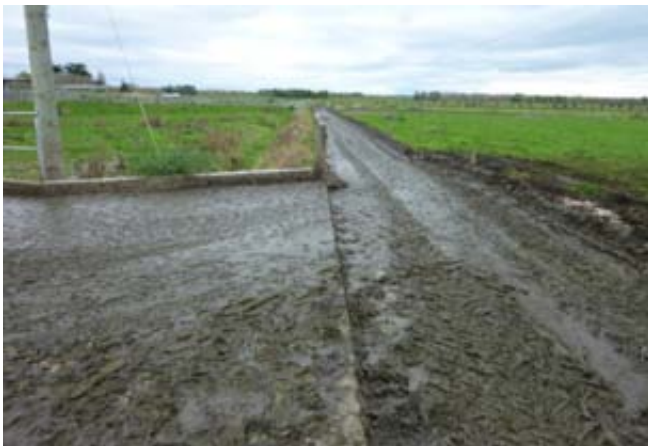
Before: Sloppy track - sloping towards drain.
