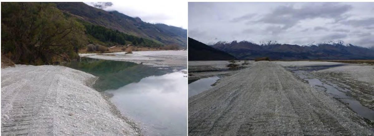
Figure 2. Temporary erosion protection works on the true right of the Dart River where the Kinloch road is at risk of erosion. See Figure 3 for location.
