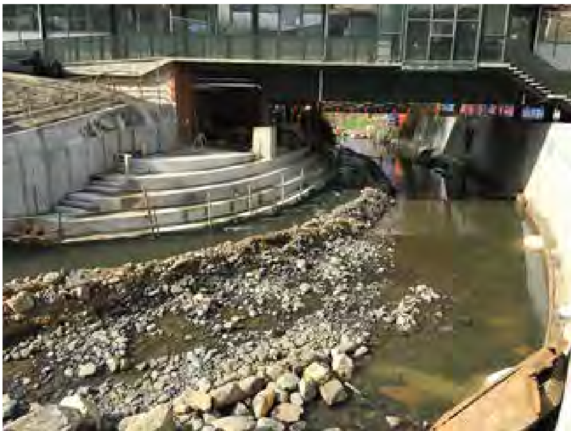
Figure 4. Looking downstream along the bed of the Water of Leith towards the Information Technology Services (ITS) Building (4 September 2018). Works are being undertaken below the ITS building and the river is temporarily diverted adjacent to the left bank wall.
