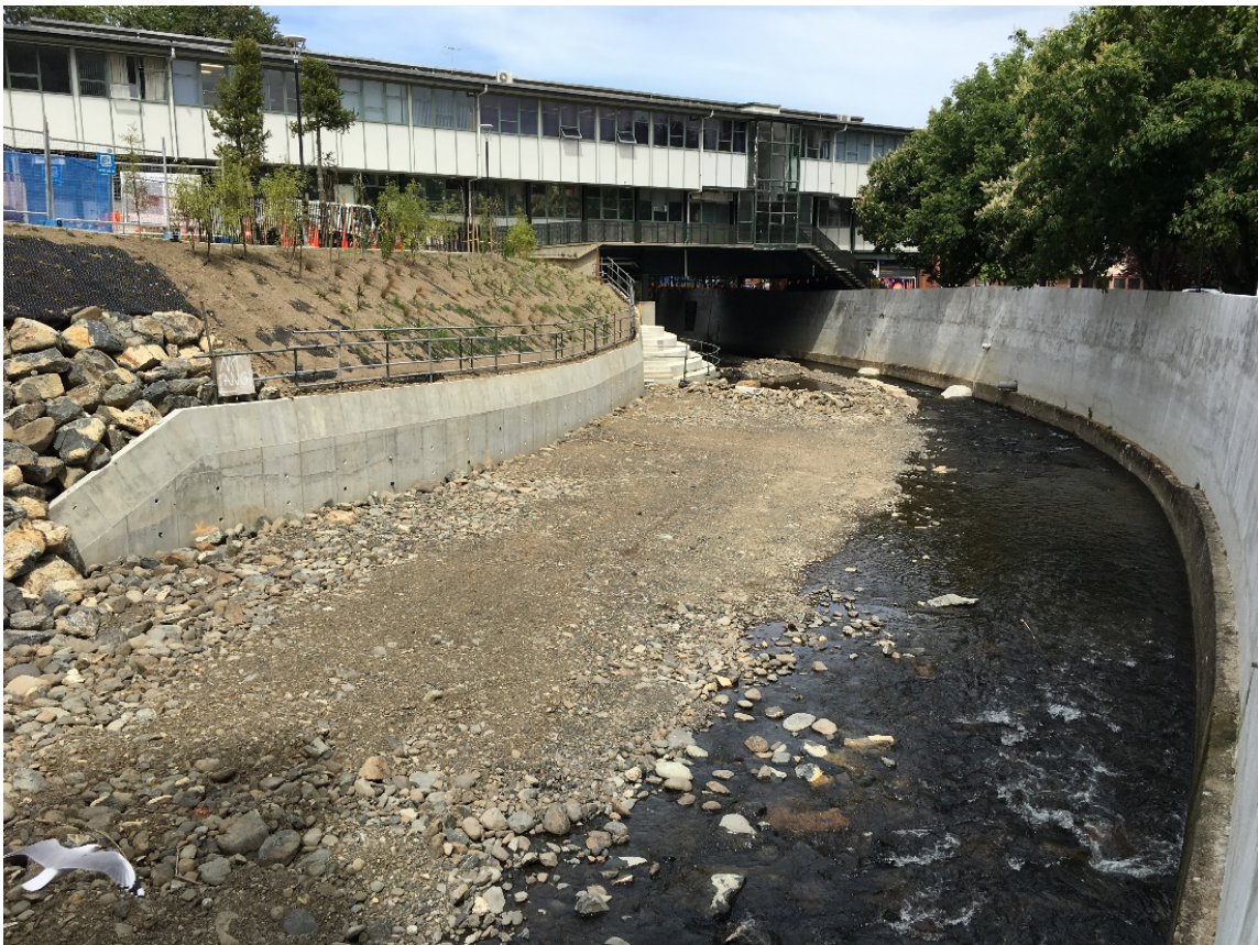
Figure 8. Looking downstream along the bed of the Water of Leith towards the Information Technology Services (ITS) Building (14 November 2018). River flows have been temporarily diverted to the right.
