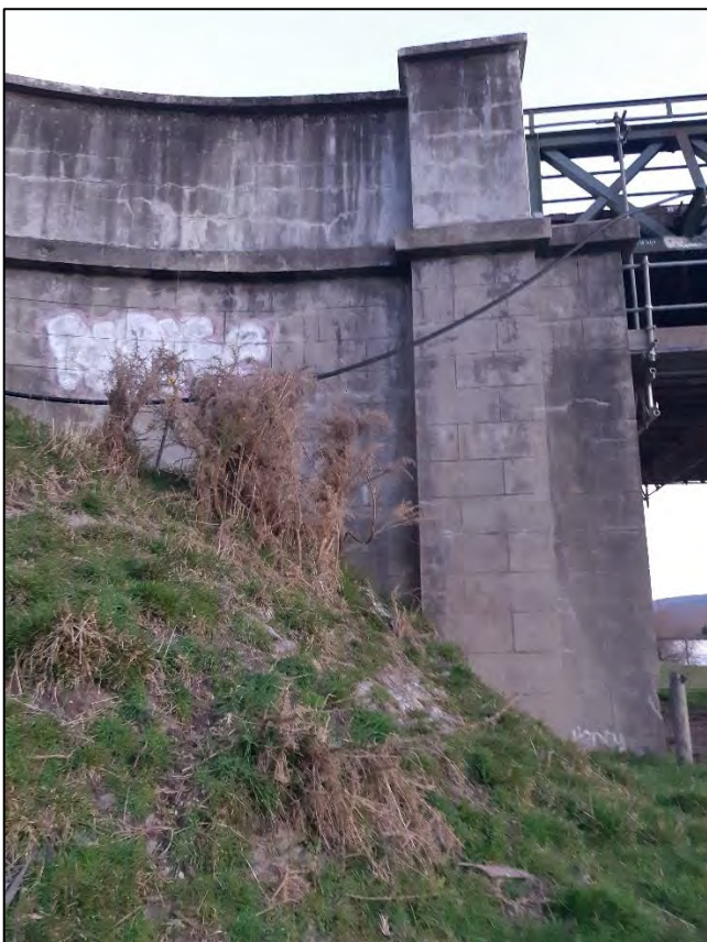
Figure 22. View looking south of the eastern Beaumont Bridge abutment, showing the built-up bridge approach in foreground
