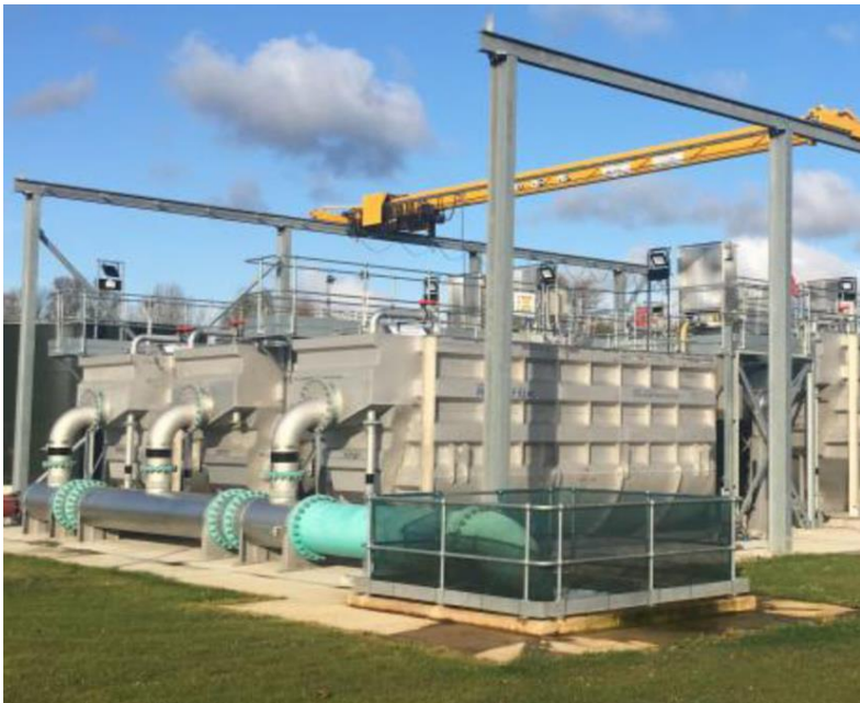
Figure 13 Example figure of tertiary filter installation (online photo, from WaterProject)
