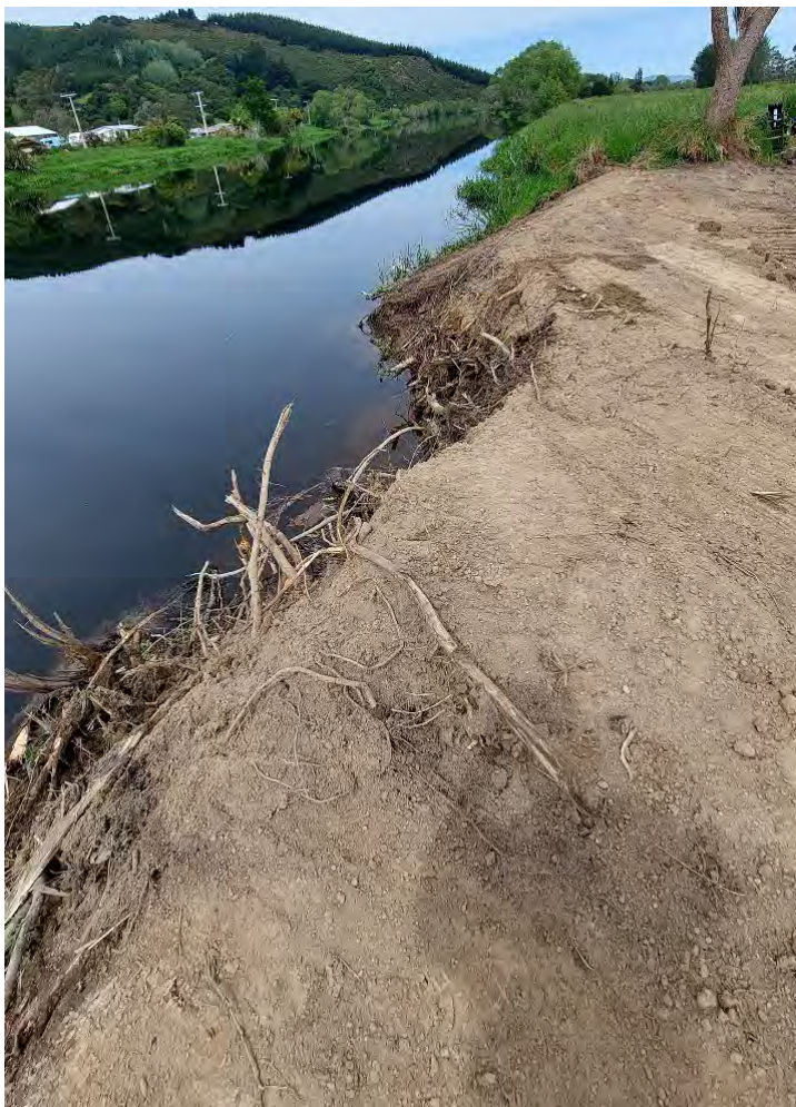
Figure 6. Bites taken out of the floodbank following the 2024 event.
