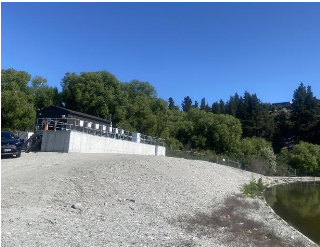
Figure 8 UV system, located at the back end of Pond 3, photo taken at the transfer pumps, November 2024.
