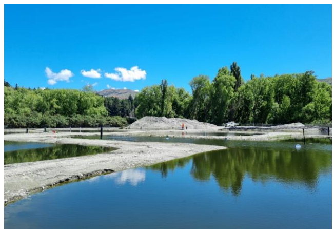
Figure 4 Disposal field now acting partially as a RIB system, photo taken by GHD in Nov 2024.
