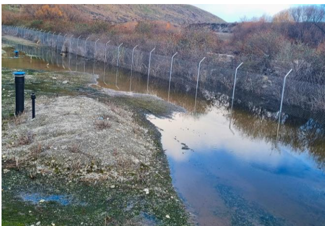
Figure 3 Ponding and surface runoff near the disposal field, 2022, photo provided by QLDC.
