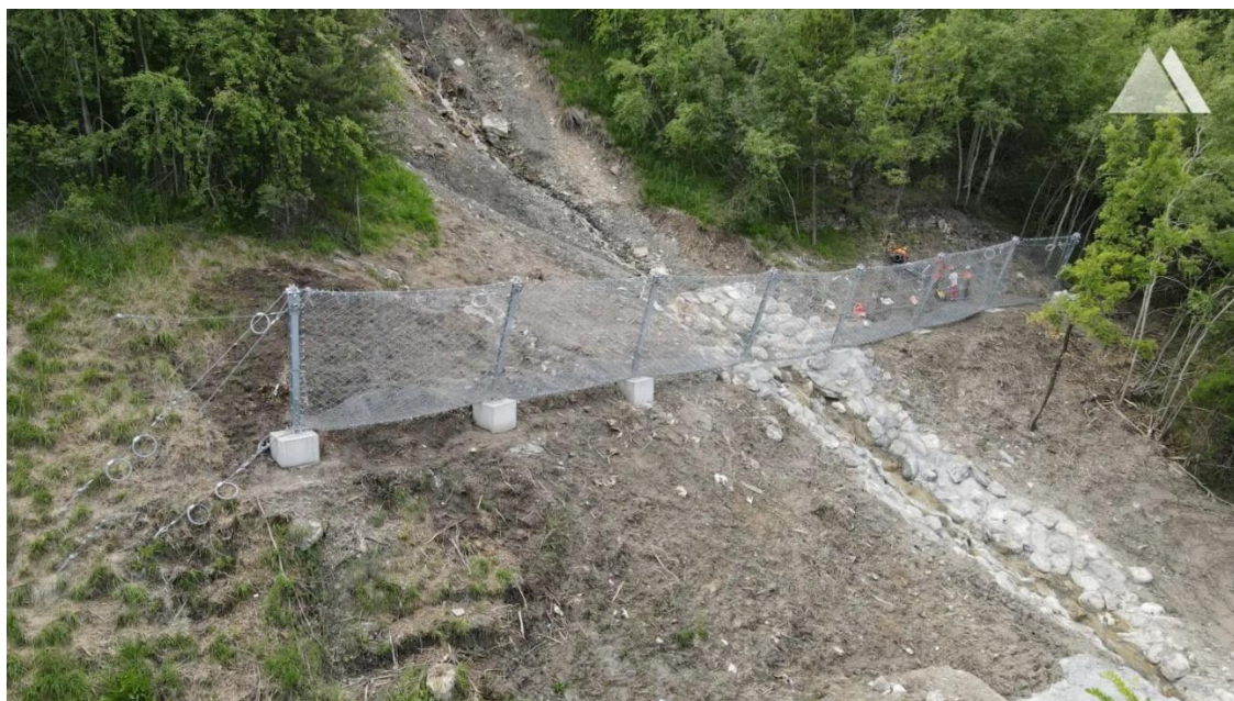
Figure 7: A Geobrigg debris flow barrier in Reotier, France (credit: Geobrigg).
